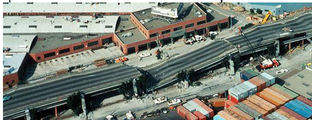
Collapsed sections of the Nimitz Freeway. Photo by H. G. Wilshire for US Geological Survey.
